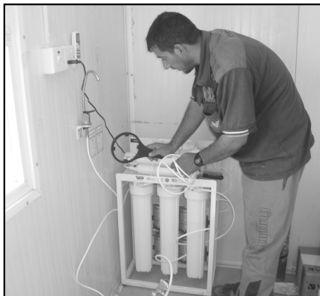
An installed water sterilizer and filtration near Nassiriya
